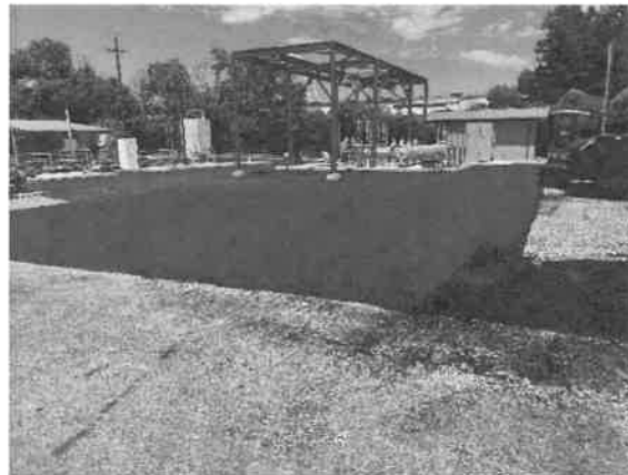
Paving Day 2 – Contractor paves remainder of site. Paving was completed around the north side of the electrical building as well.
