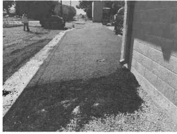
End of Day 1 for asphalt paving. Contractor finished northwest end of the site by the Auxiliary Headworks and the electrical building.
