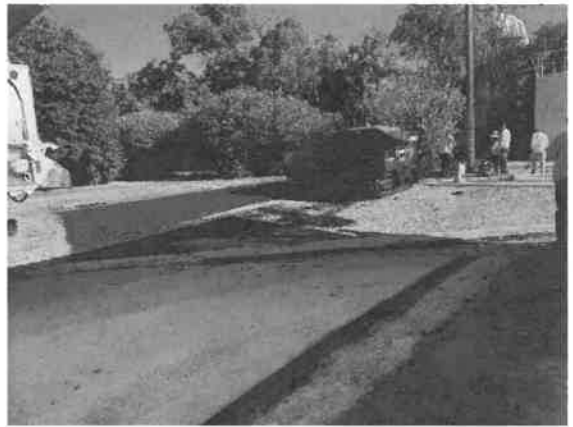
Edges of existing pavement were coated in tack coat and Contractor began to lay asphalt.
