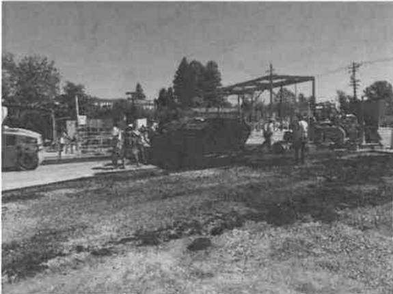
The Contractor lays asphalt paving the south side of the site near the wet well and vaults.
