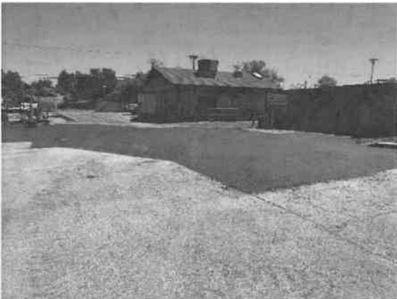
End of Day 1 for asphalt paving. Contractor paved driveway and around vaults.
