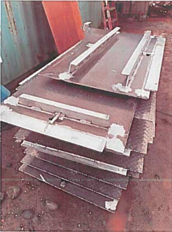
The Contractor trims and grinds the aluminum plate covers for the influent screening facility.
