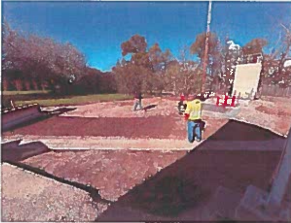
The Contractor lays and compacts AB around the HRS Flowmeter Vault and Flow Control Vault.
