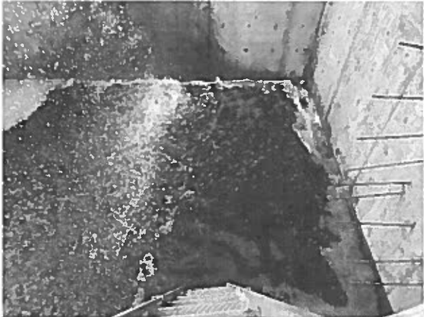
The wet well was filled with water to conduct the watertightness test.
