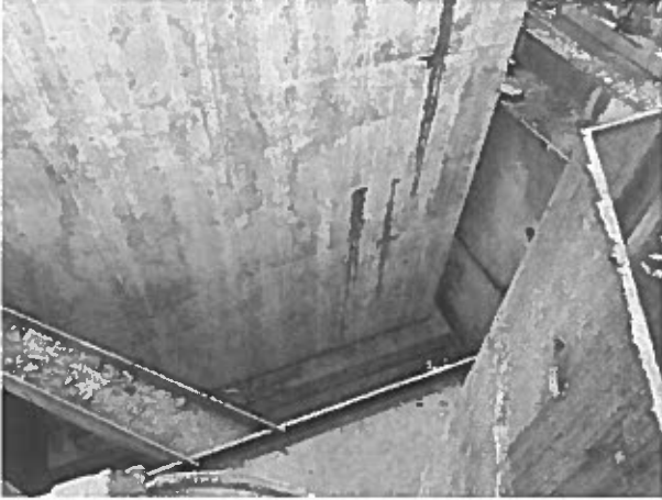
Several leaks were discovered at various locations on the exterior of the structure during water tightness testing.
