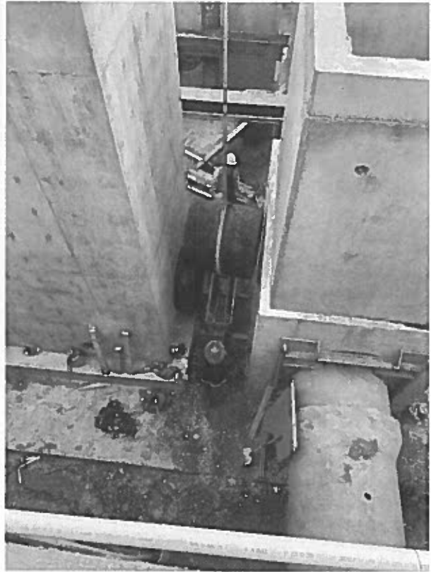
36" ductile iron pipes were placed between the Bar Screen Structure and both Diversion Box structures.
