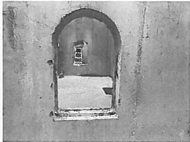
The 18" pipe penetrations in the north and south walls of the precast metering vault structure were lowered by sawcutting through the concrete and rebar.
