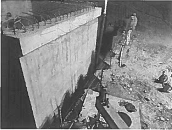
The Contractor partially backfilled the wet well area with slurry after successful watertightness testing.
