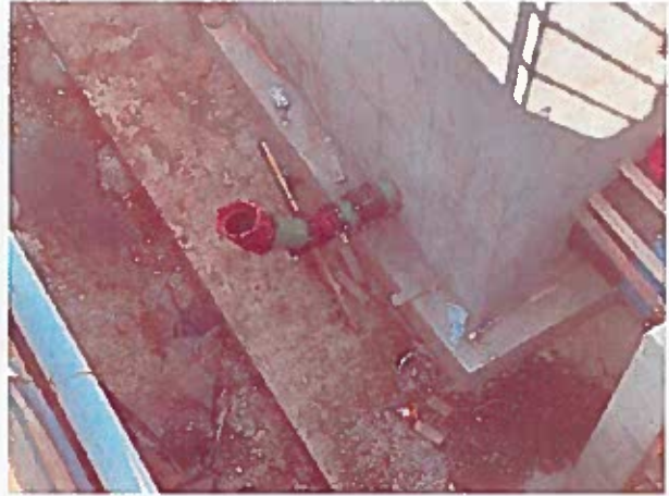
The Contractor installed the bar screen structure sample access port and sealed the annular space with grout.
