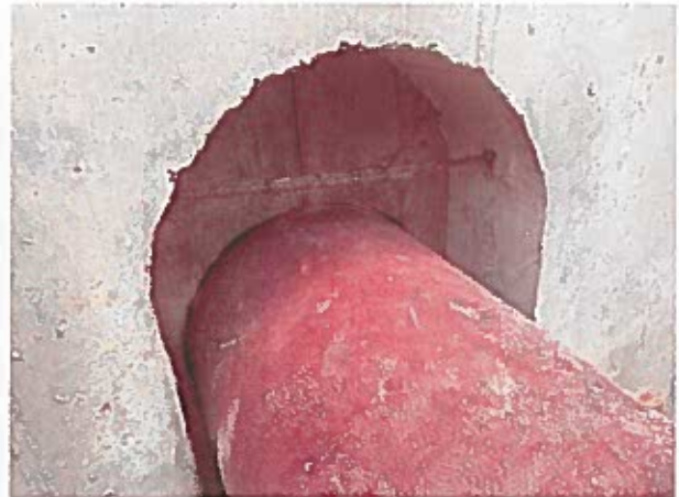
The Contractor installed rebar inside pipe penetrations that was cut to lower the pipe penetrations through the metering vault.
