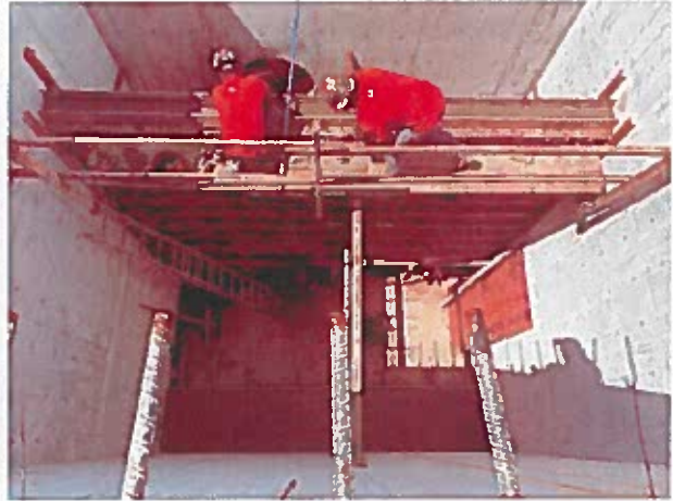
The baffle wall and pump pedestals inside the wet well were poured.
