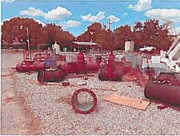
The Contractor assembles pipe outside of the excavation to be lowered into the vaults with a crane.
