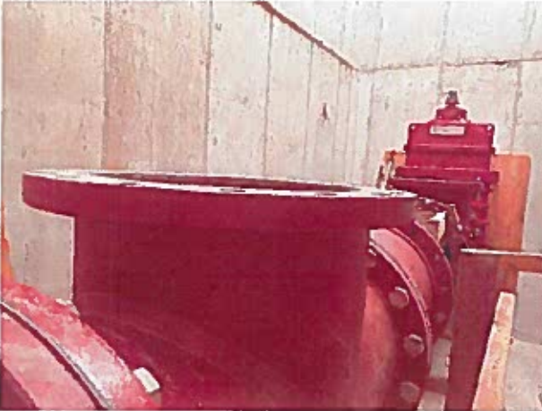
Piping, fittings, and knife gate valves were installed in the metering vault.
