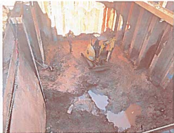
Proposed Wet Well location excavated below influent manhole bases to proposed base grade and saturated with groundwater.
