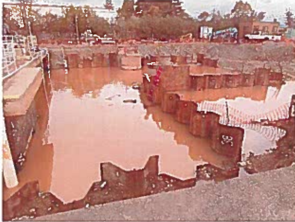
Excavation is flooded after storms with groundwater.
