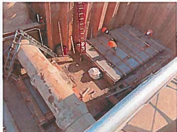
Concrete is poured in the vault base of Diversion Box 2 and Metering Vault.
