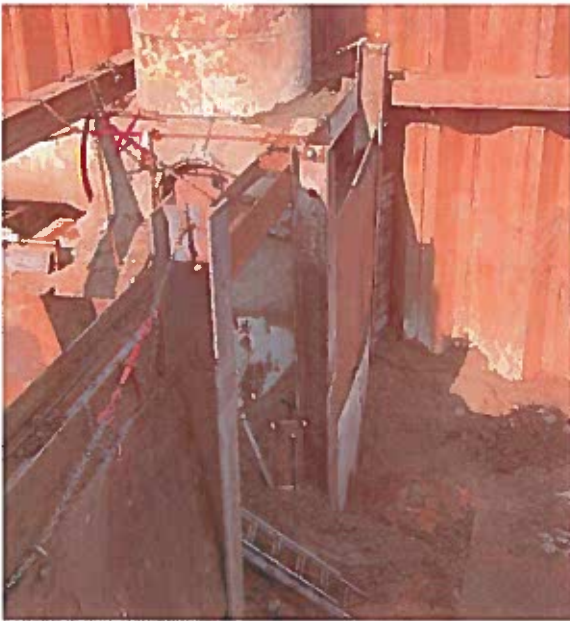
Slurry was poured between existing manhole structure and shoring plates to stabilize the foundation of the manhole after undermined soil was observed.
