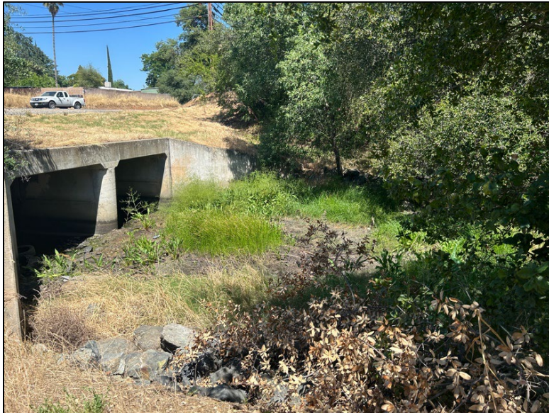
Figure 8 - View of Ruddy Creek looking northwest from western side of pump station
